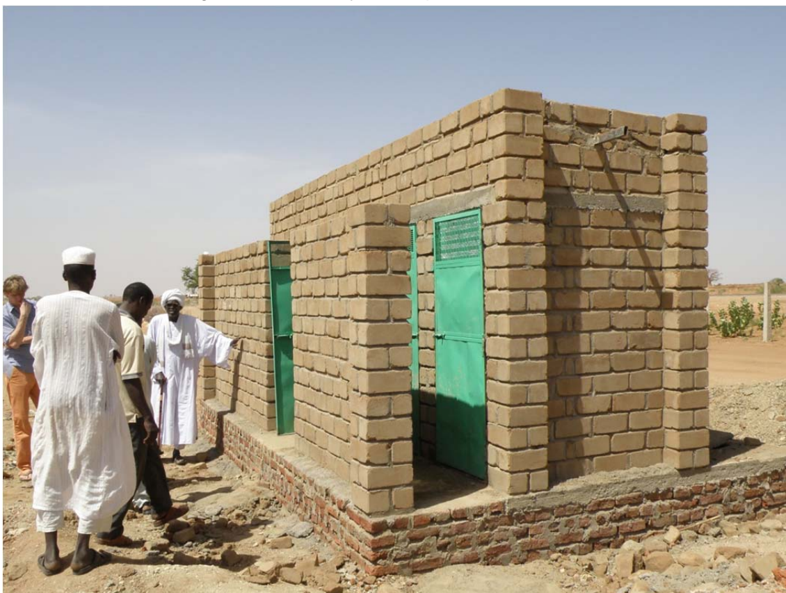
Permanent latrine for a school
